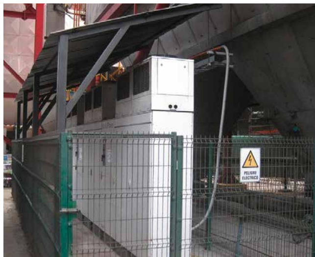
Fig. 1 AES Norgener U1 ModuPower™ lineup consists of 2 x 120kW and 1 x 150kW units. The units were installed at ground elevation with 150ft. HV cables run to ground switches on the ESP roof. Courtesy: AES Gener, Norgener Plant
