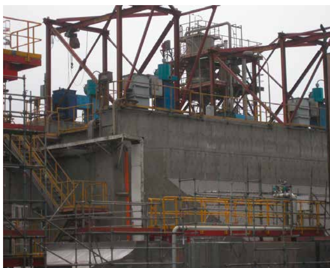
Fig. 2 AES Norgener ESP with ModuPower™ ground switches (teal color) installed on top of its ESP. Courtesy: AES Gener, Norgener Plant
